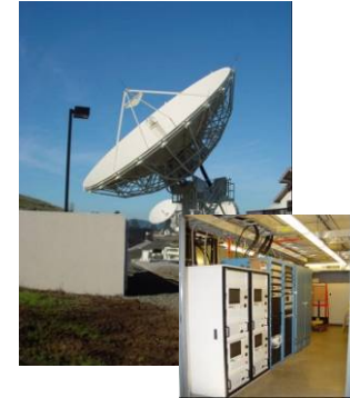
4 Ground Earth Stations
