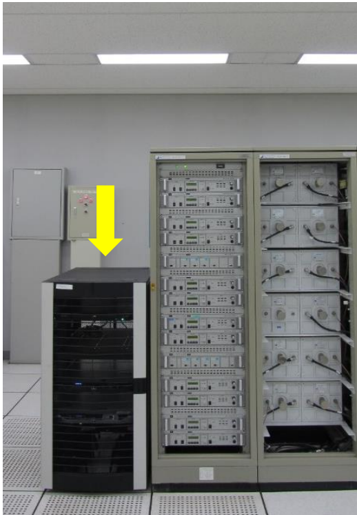
Central Processing Station
