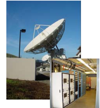
4 Ground Earth Stations
