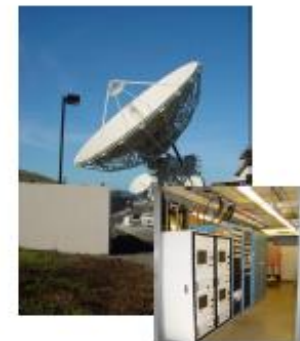
4 Ground Earth Stations
