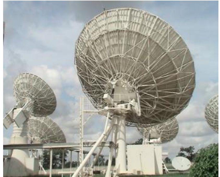
NIGCOMSAT Master Control Station with C-L Band Antenna Systems
