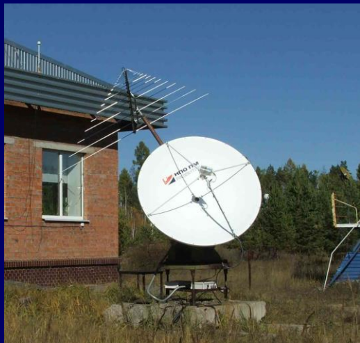
Antenna attached to dish
