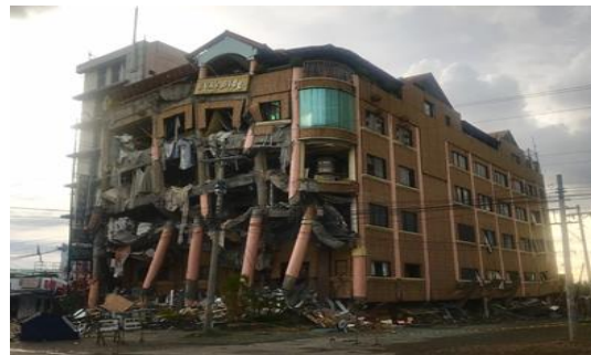
Eva's Building damaged during the October 31 2019 M6.5 event
