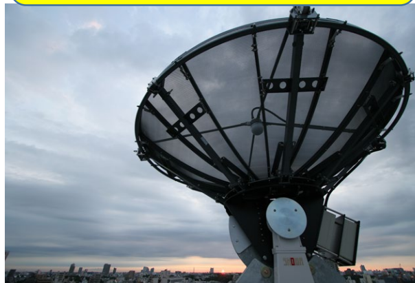
UHF/VHF/S-band Ground Station Antenna
